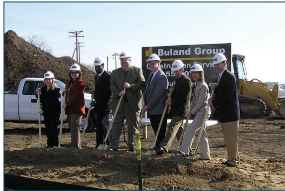
Above: Thomas Judds along with others prepare to break ground at Greenview Estates, LLC located in Omaha, NE.
