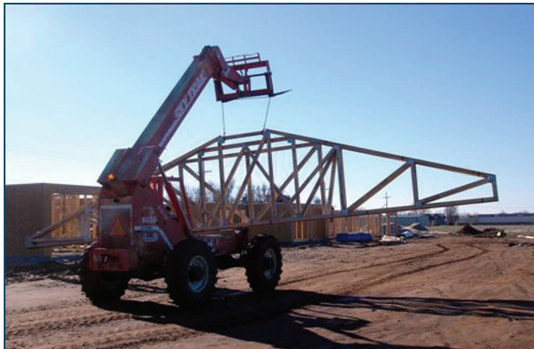
Above: Construction is underway for Sunrise Ridge Townhomes, LLC, which was recently closed in January.
