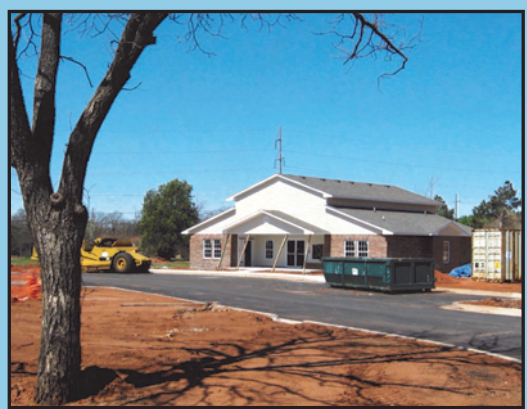
Above, construction at Mt. Olive, L.P. in Oklahoma City moves forward, despite the temperamental spring weather.
