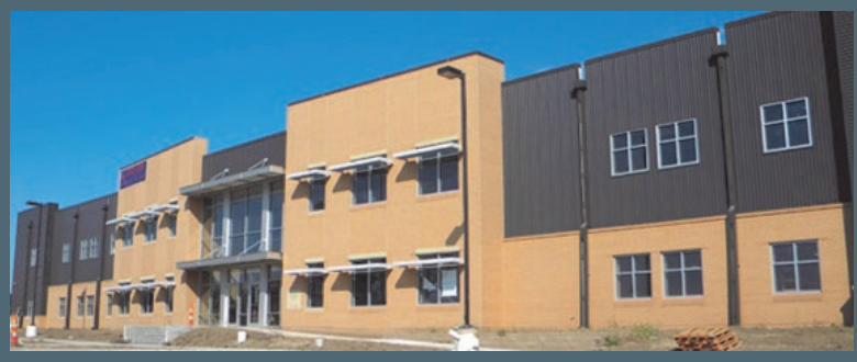
Above: The new Lydia House, part of the Rebuilding Lives campaign through the Open Door Mission, nears completion. Once open, the Lydia House will provide 36 single women beds and 46 family units for those in need in the Omaha metro.
